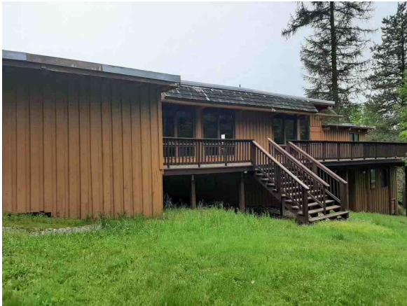
rear, deck in fair to poor condition
