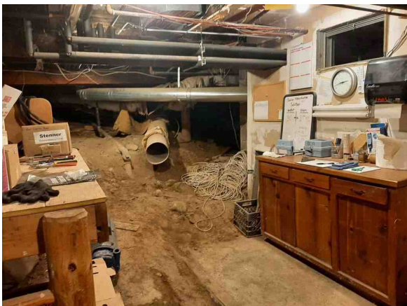
water filtration system in lower level of Mare's Lodge
